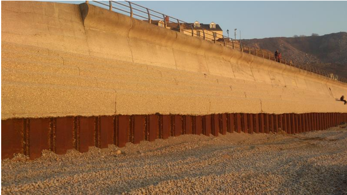
Figure 19 - flood defence sea wall on Chesil Cove Beach, Dorset (BennH, 2014, https://commons.wikimedia.org/wiki/File:Chesil_Cove_flood_defences.png [unedited]).
