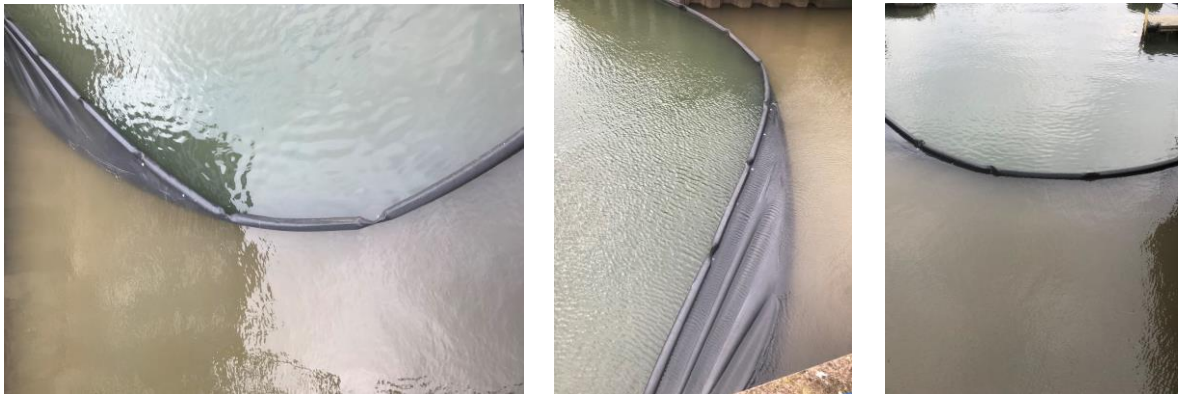
Figure 4.1: Photos demonstrating silt curtain at Exmouth Marina entrance during dredge operations (Source: Lewington and Irwin, 2018)
